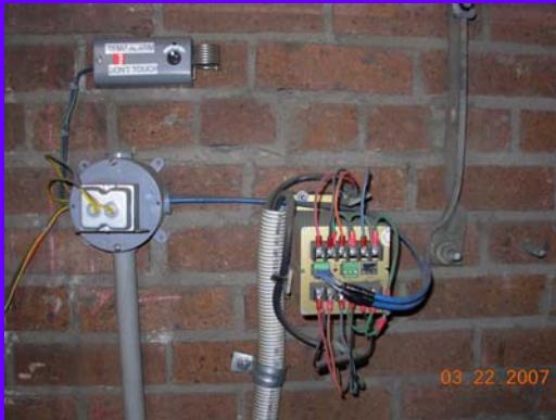
IQ200 Meter to Monitor Street Feed Load
