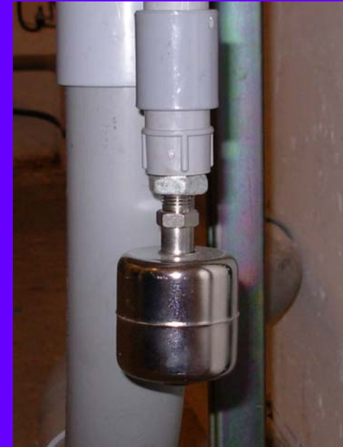
Float Switch Connected to Digital Input Module
