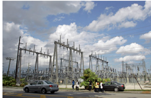
A substation located next to Florida Power and Light headquarters is shown in Miami, Tuesday, February 26, 2008. Florida experienced a widespread power outage on Tuesday.
